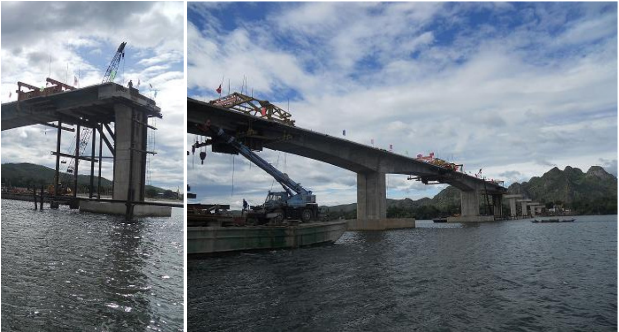
Bridge and road to Van Hoa commune, Tuyen Hoa District, Quang Binh Province ..... Balanced cantilevered pre-stressed concrete structure
