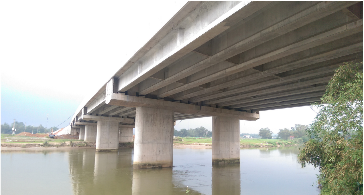
Package 01: Km0+00 Km8+00 LRB02 Bridge Km02+460.75 across Yen River – Danang City Pre-stressed concrete structure L=33m
