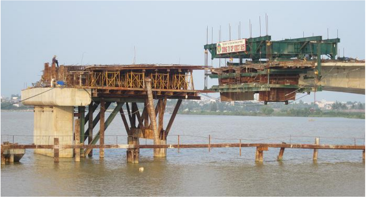
Road Project connecting Hoa Xuan Bridge and Hoa Quy ecological urban area ..... Balanced cantilevered pre-stressed concrete structure
