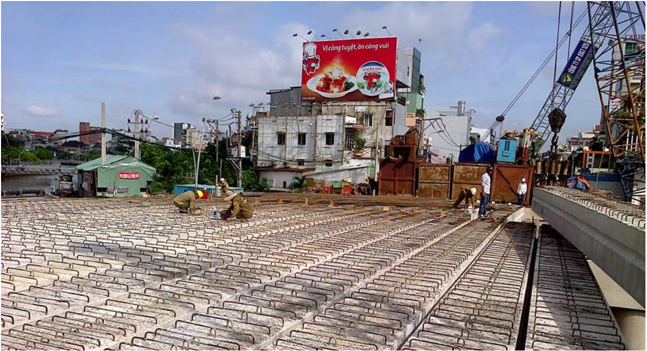
Project for Construction of 4 Bridges: Le Van Sy Bridge, Kieu Bridge, Bong Bridge on Nieu Loc - Thi Nghe canal Hau Giang Bridge on Tan Hoa - Lo Gom
